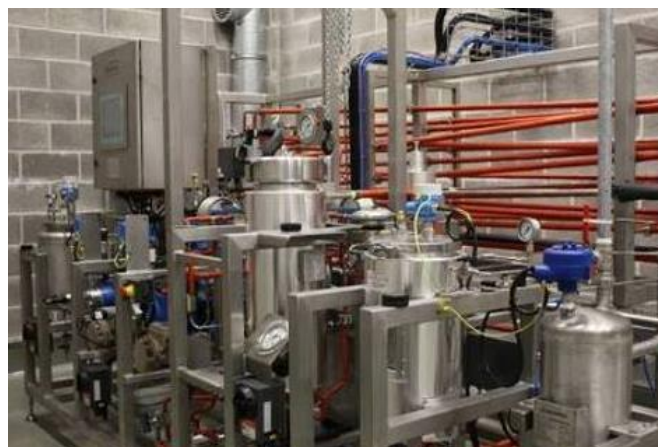
Subcritical water extraction pilot plant at the CELABOR facility
